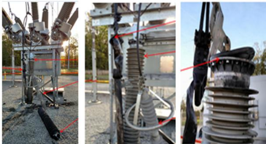
Figure 27 - Failed Station Equipment
