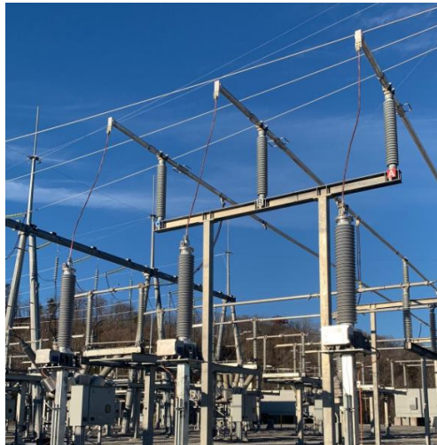
Figure 11 – Three RC voltage dividers at a 161 kV TVA substation
