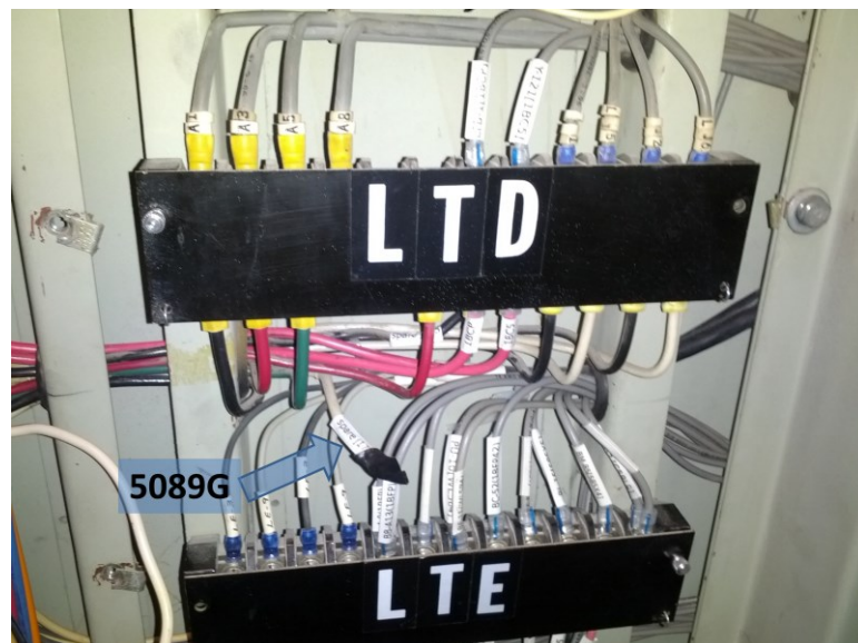
Figure 8. Lifted residual wire in 5088 CT circuit to feeder differential circuit (first terminal block in control building).
