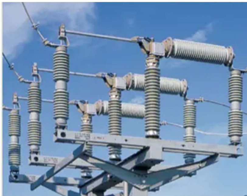
Figure 6: Horizontal interrupter circuit switcher with integral vertical disconnect switch
