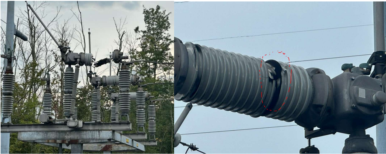
Figure 2: the damaged 115kV circuit switcher CS-1 and cracked housing on B-phase interrupter
