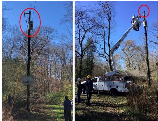
FIGURE 6 LOCATION OF CRACKED INSULATOR AND DAMAGED TRANSFORMER
