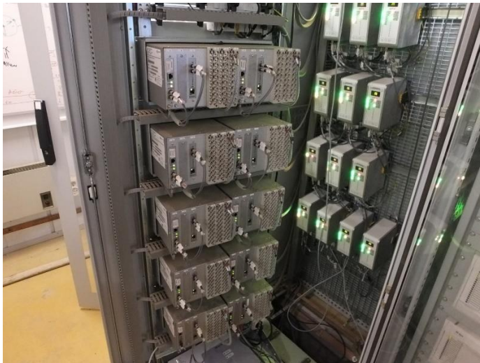
Fig. 2 Multifunctional IEDs in a digital substation
