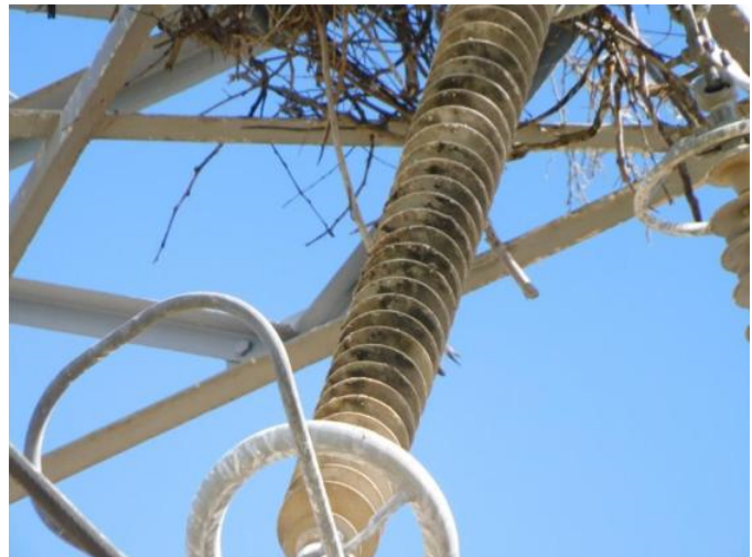
Fig. 11. Evidence found of the December 17, 2019, fault, showing bird contamination and arcing across the insulators.
