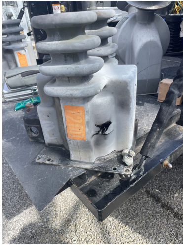
Figure 8. Failed VT at Albertville
