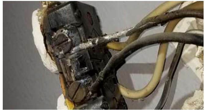
Figure 2 - Damaged Wall Outlet
