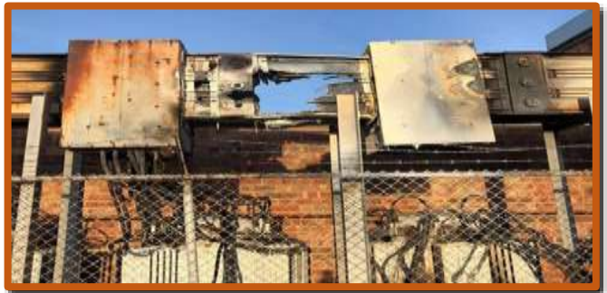
Figure 6 - Burned Bus work
