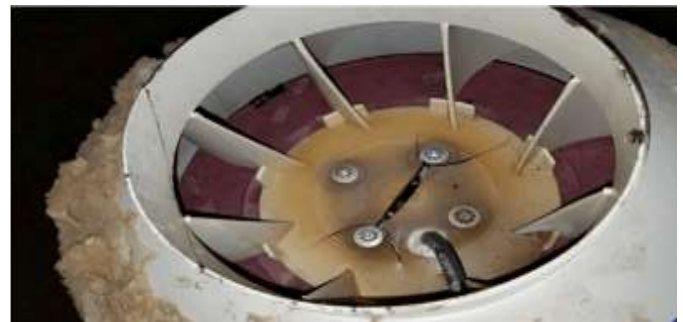
Figure 3 - Failing Radon Pump
