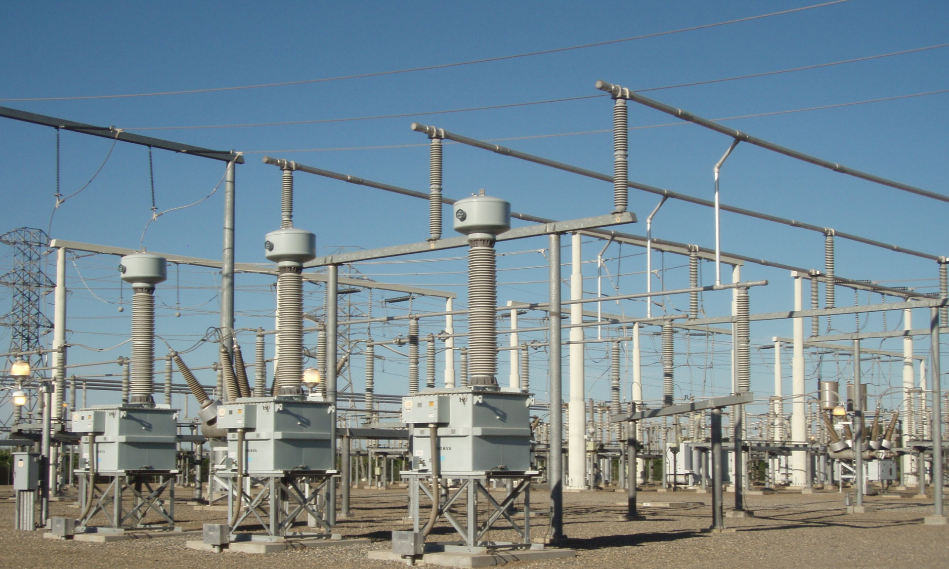
GREGG 230 KV SHUNT REACTOR BANKS 100 MVAR
